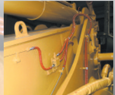
Pipe work protected with special heat shield shrouding
