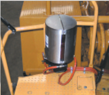
Pump reservoir fitted with metal protection shield
